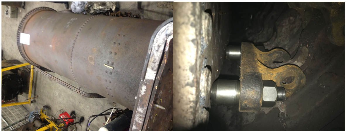
Left: Boiler barrel with smoke box end to the left. Right: New crown stays(sideways on boiler top is to right).
